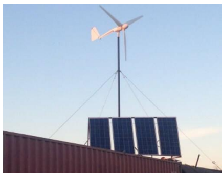
Fig. 1. Photograph of the experimental hybrid wind-solar power plant
